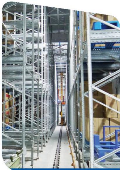
货架系统 Racking System
