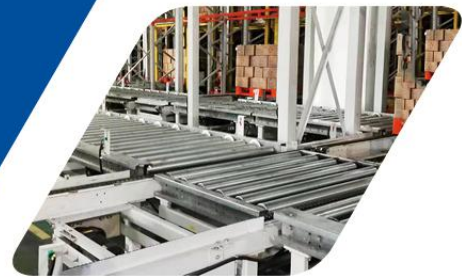
输送系统 Conveying system
